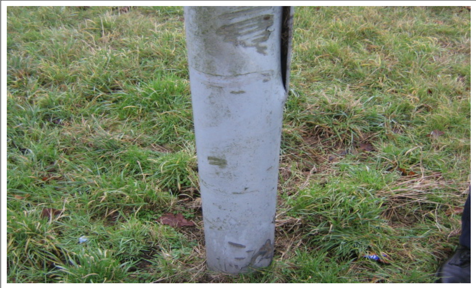
P0003 – Grey paint / coating to older lamp post at Sherbourne road
